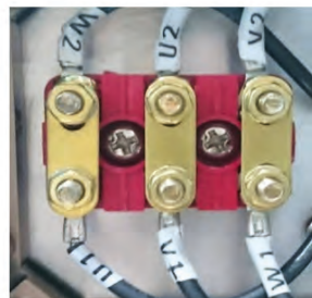
230V three-phase connection
