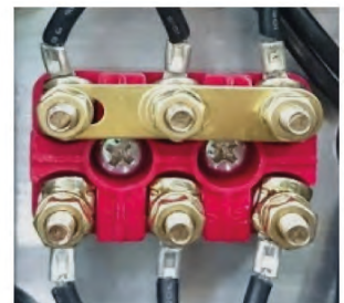
400V three-phase connection
